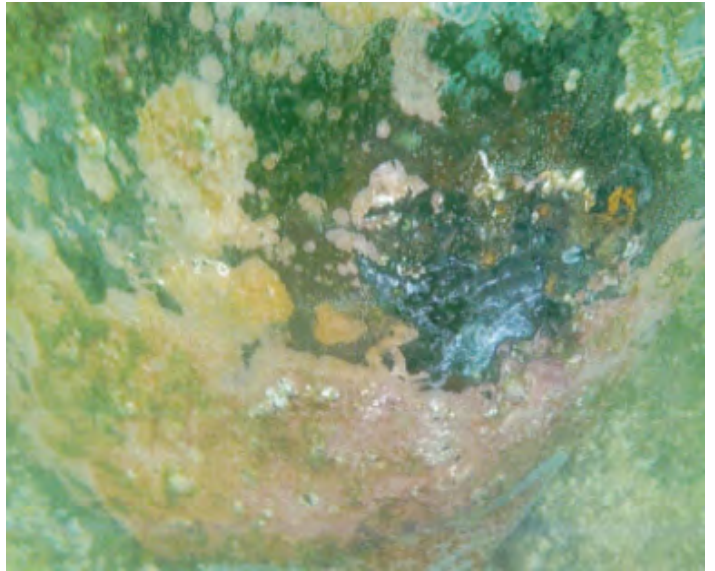
Photo 40: SP4-B deep pitting
