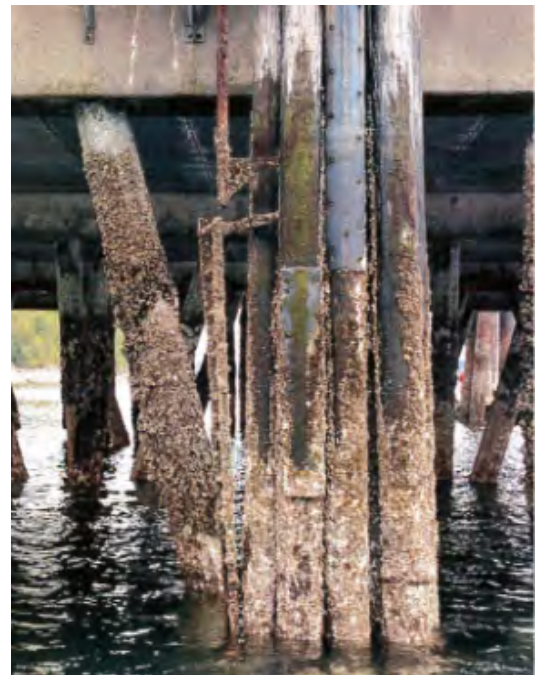
Photo 66: Dolphin D2 with abrasion damage, ladder detached
