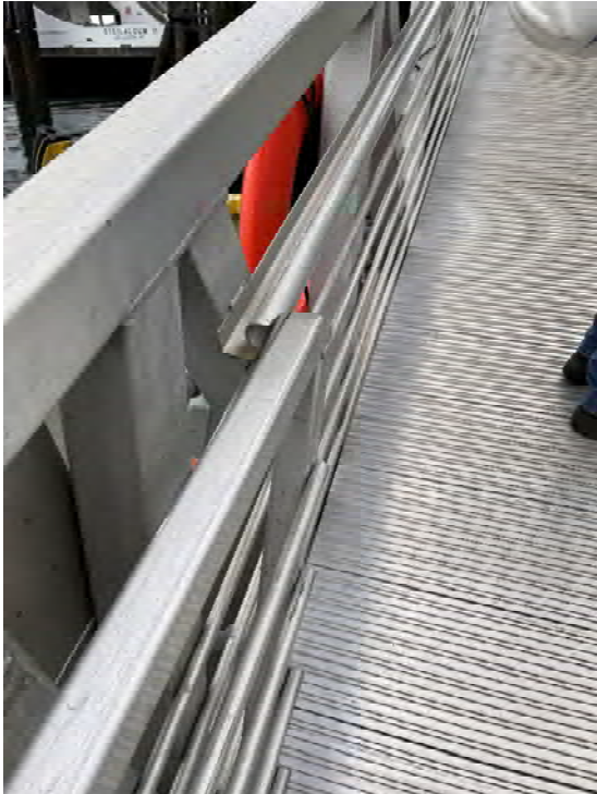
Photo 21: Loading ramp handrail with sharp edge
