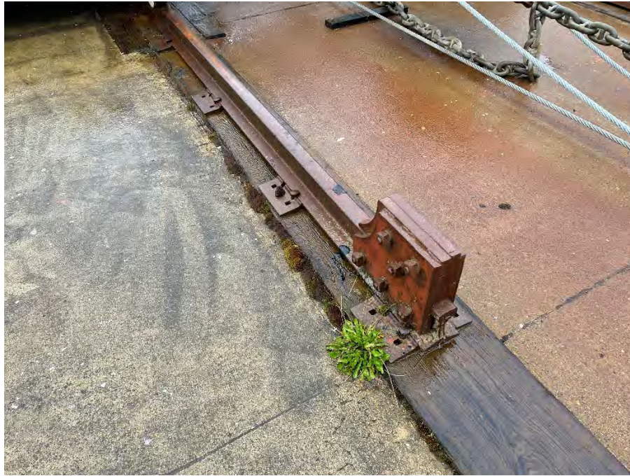
Photo 126 : Surface corrosion on rail North of bulkhead
