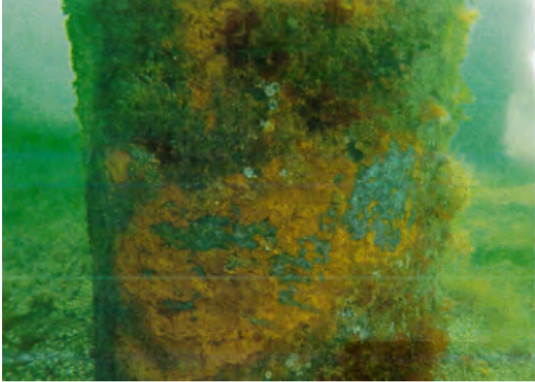
Photo 34: SP4 coating failure and surface corrosion
