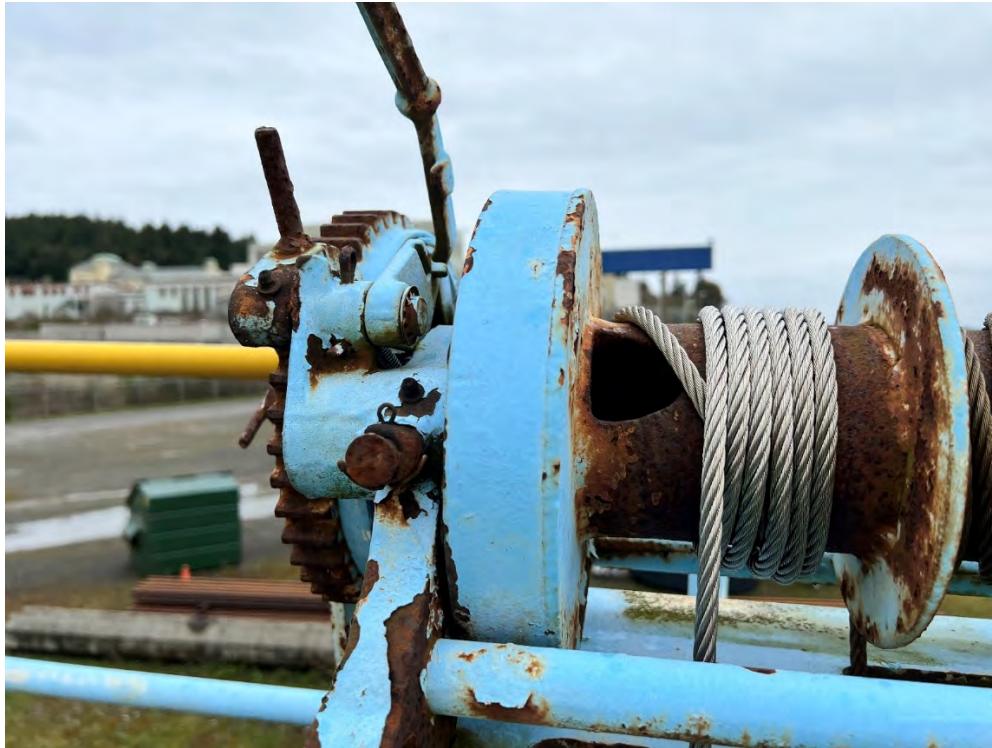
Photo 189: Bilge block hand winch
